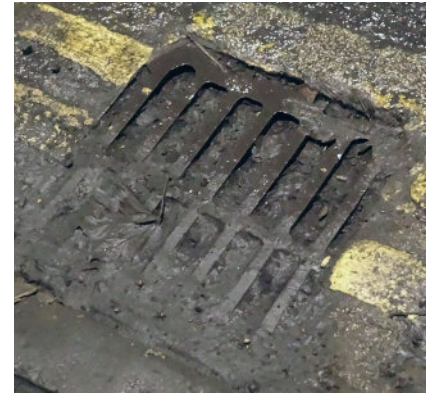
adequately maintain existing drains
